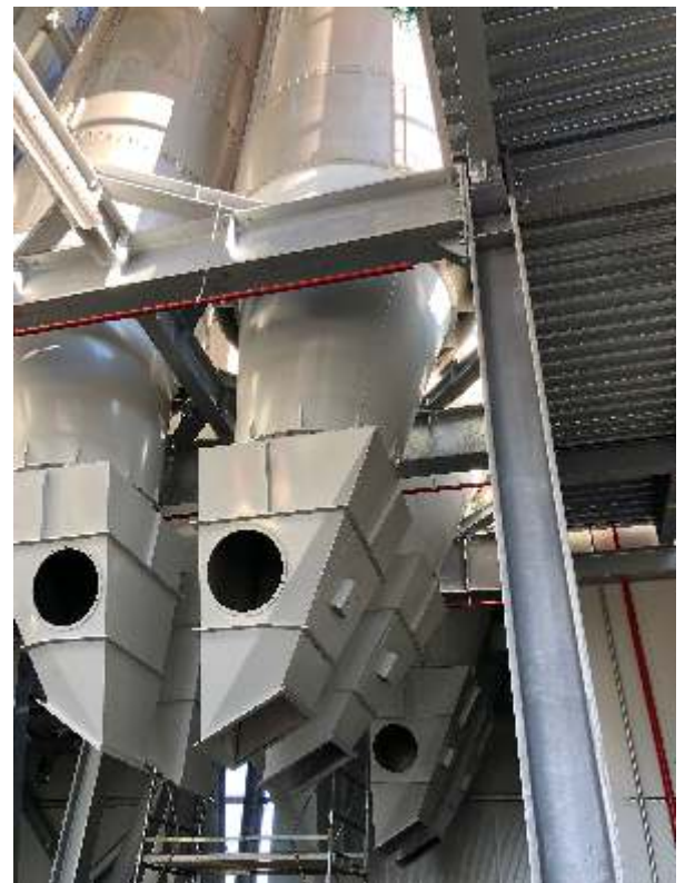
Smooth bolted silos with asymmetrical hopper for bulk trucks load.
