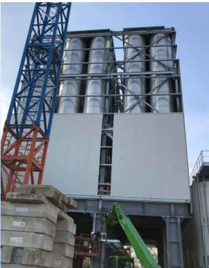
Stainless steel bolted silos, arranged in battery, on a metal structure.
