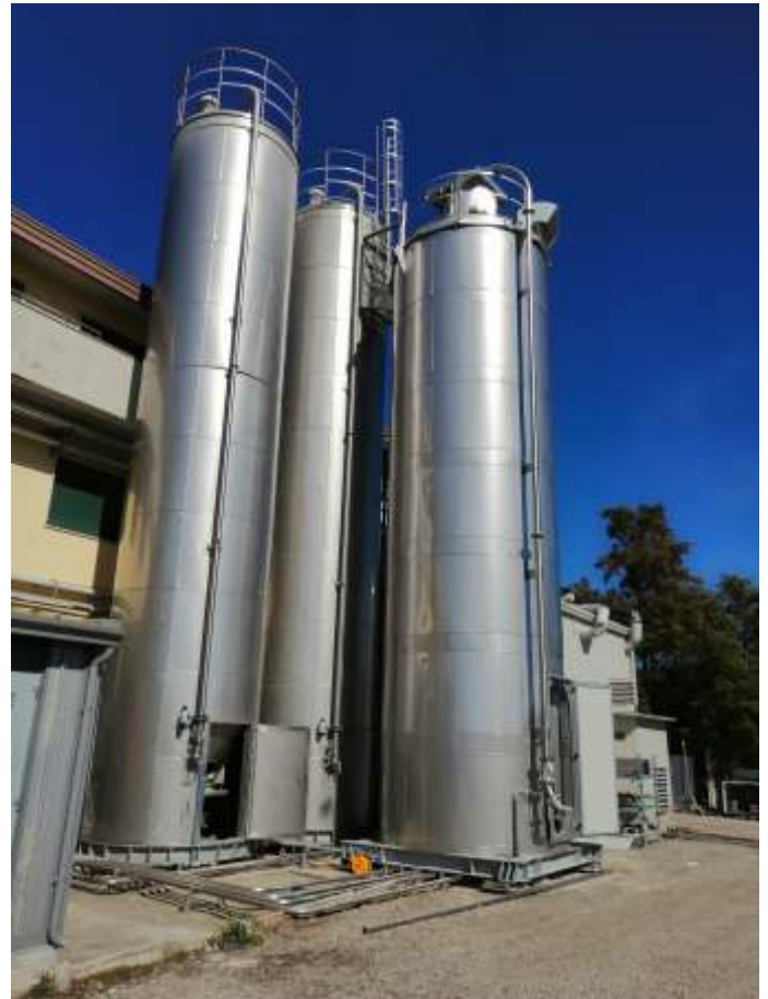
Stainless steel bolted silos, on a skirt solution, individually insulated, for tanker unloading.
