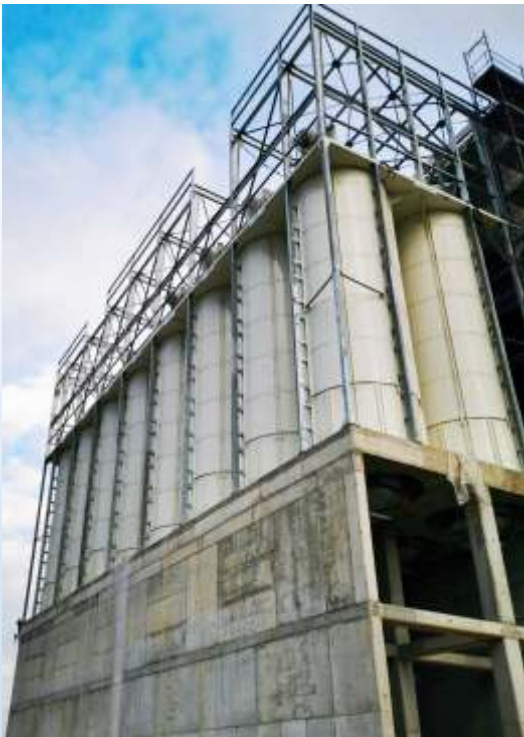
Powder coated smooth bolted silos, arranged in battery, on a reinforced concrete structure.
