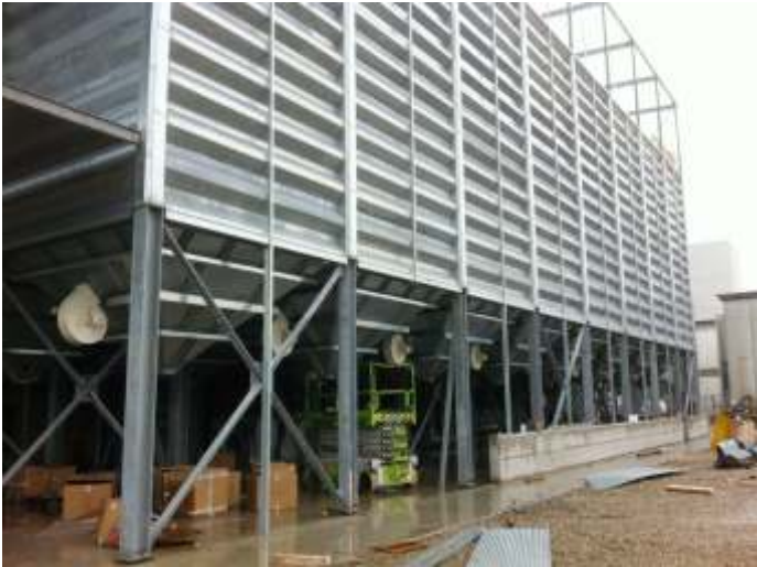
Flat wall cells battery, corrugated type, on a metal structure.
