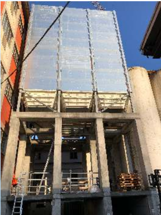
Flat wall cells battery, smooth sandwich-type, on a reinforced concrete structure.
