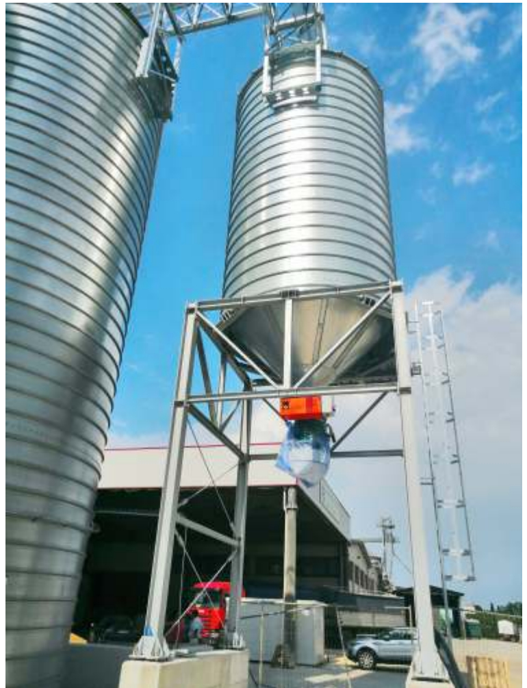
Hoppers smooth spiral silo, on a metal structure for bulk trucks load.
